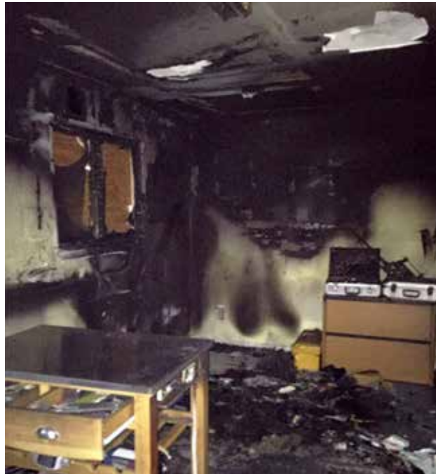
This fire was started by a small 3S lipo that would not normally be considered dangerous.
