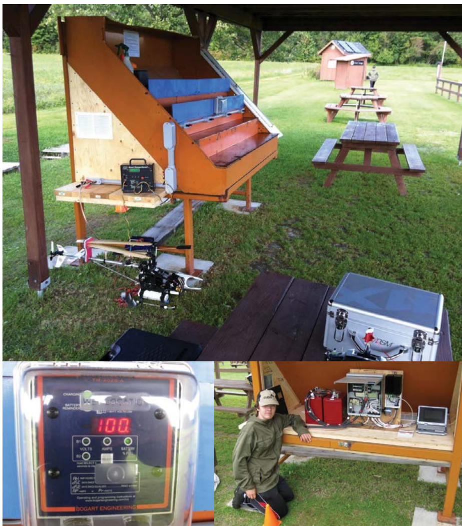
Top: The charging station can be seen in the front while the solar panels can be seen on the utility shed in the background. Bottom left: The 'solar battery' capacity meter. Bottom right: Showing off the main system components is my son Gabriel who helped out with the system installation. The portable computer was used to verify initial system performance.
